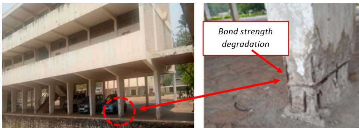
Fig. 1. Case of bond strength degradation at the base of the bearing columns of the building of the Institute of Physical Education and Sports at University of Burundi
